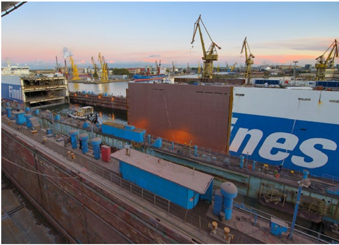
A 30-metre section was inserted between the parts and welded together. Photo: Sławomir Lewandowski
