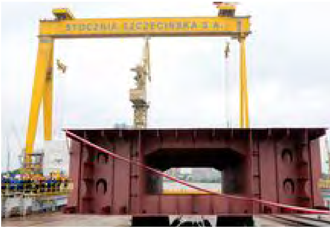
Keel laid for the construction of the new ro-pax ferry. Photo: Adrian Aleksiewicz
